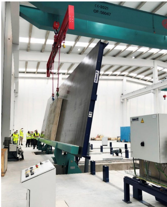
Image 6: A lifting beam is used to remove the walls from the tipping station and place them on loading racks.
